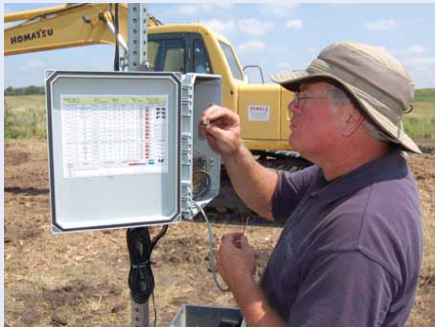
The installation of the bioreactor system is complete, and John Jordison of Agri-Drain is installing automated monitoring and sensing equipment.
