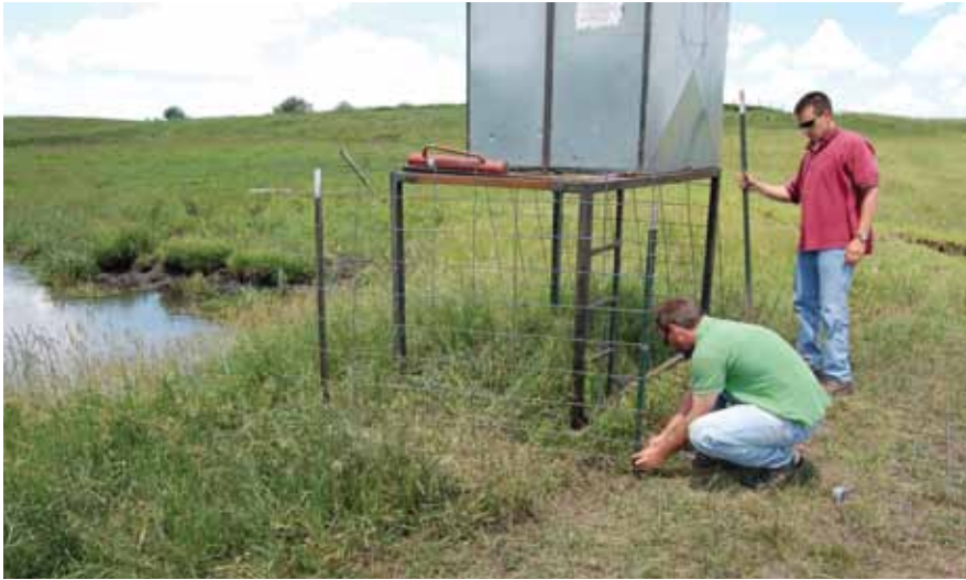
ISA staff Todd Sutphin and Anthony Seeman install an automated water quality monitor in the Boone River watershed.
